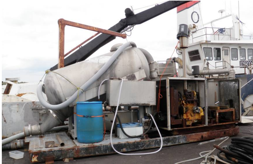
Figure 10. This pump, situated on a dock, is used to move the herring from the boat and into the dewatering box and eventually a truck or container, situated portside.
