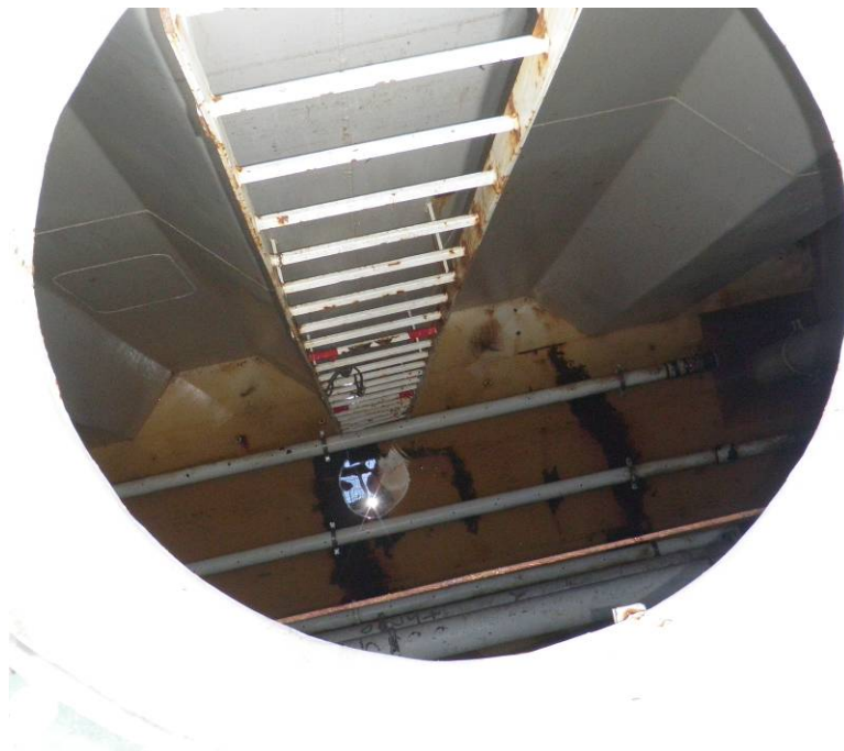
Figure 8. A holding tank, empty
